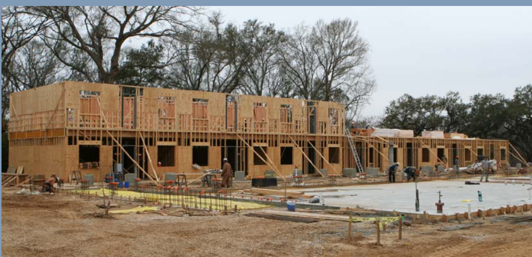
The second story and the second slab are underway. Roof coming next week!
